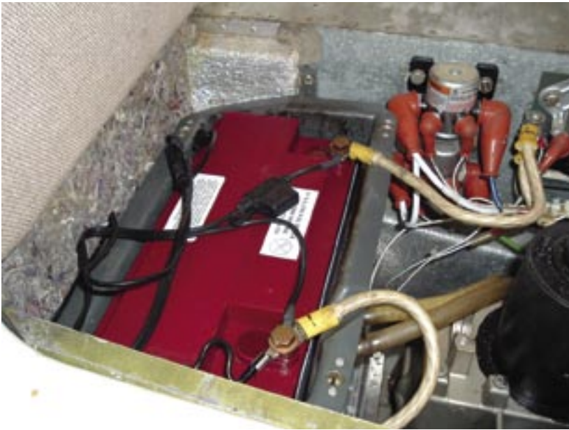
Battery Minder leads connected to battery.
