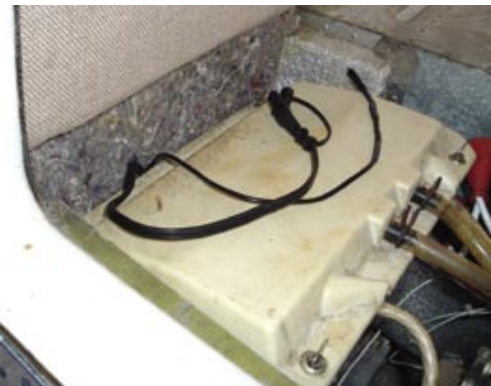
Battery Minder leads from battery cover.
